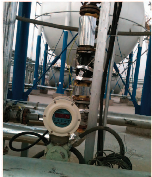
图9 VCM储罐外测液位计应用现场图片 Fig.9 VCM Live pictures outside the tank level gauge measurement applications
